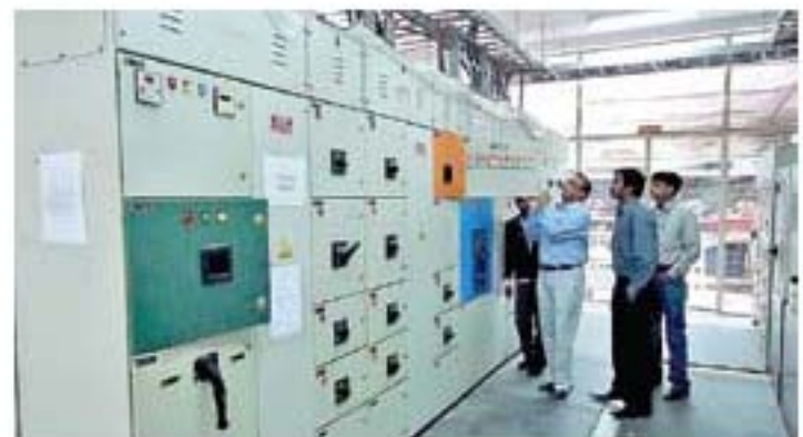
Investment Grade Energy Audit in Progress in an Apparel Industry unit in Dehi GCR
